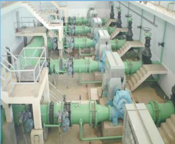
Kirloskar Butterfly, Sluice and Dual Plate Check Valves installed at Saurashtra pipeline Project, Gujarat, India
